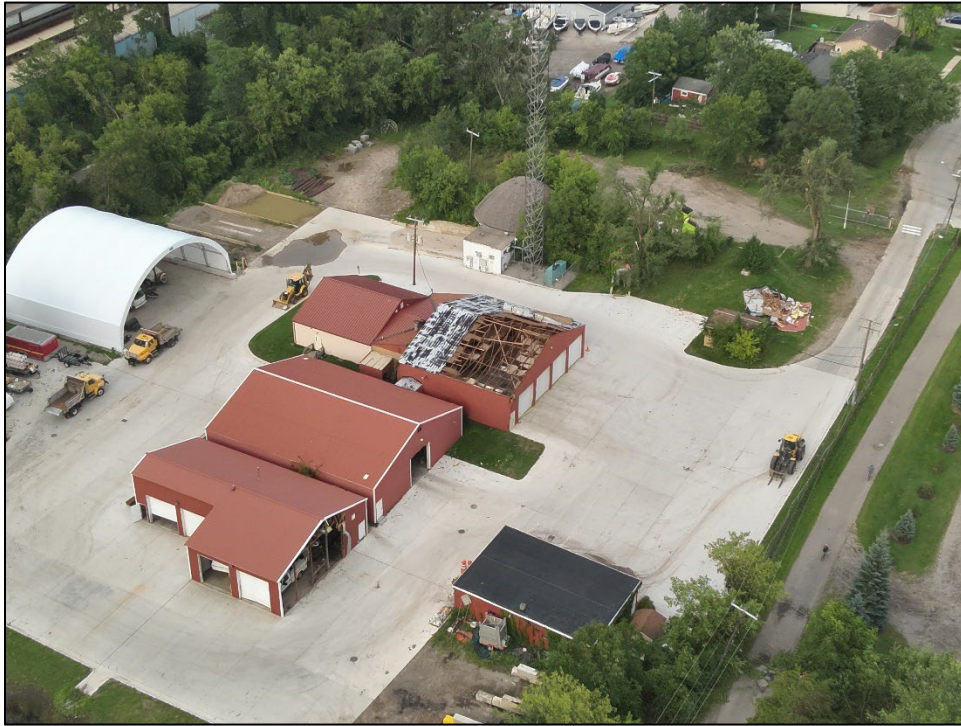
Figure 4-80. Damage from Storm
