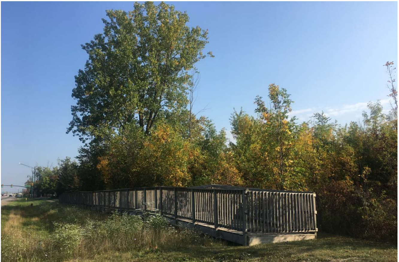
Boardwalk # 9: Dead-end boardwalk, currently closed, located east side of Beck Rd, south of Central Park
