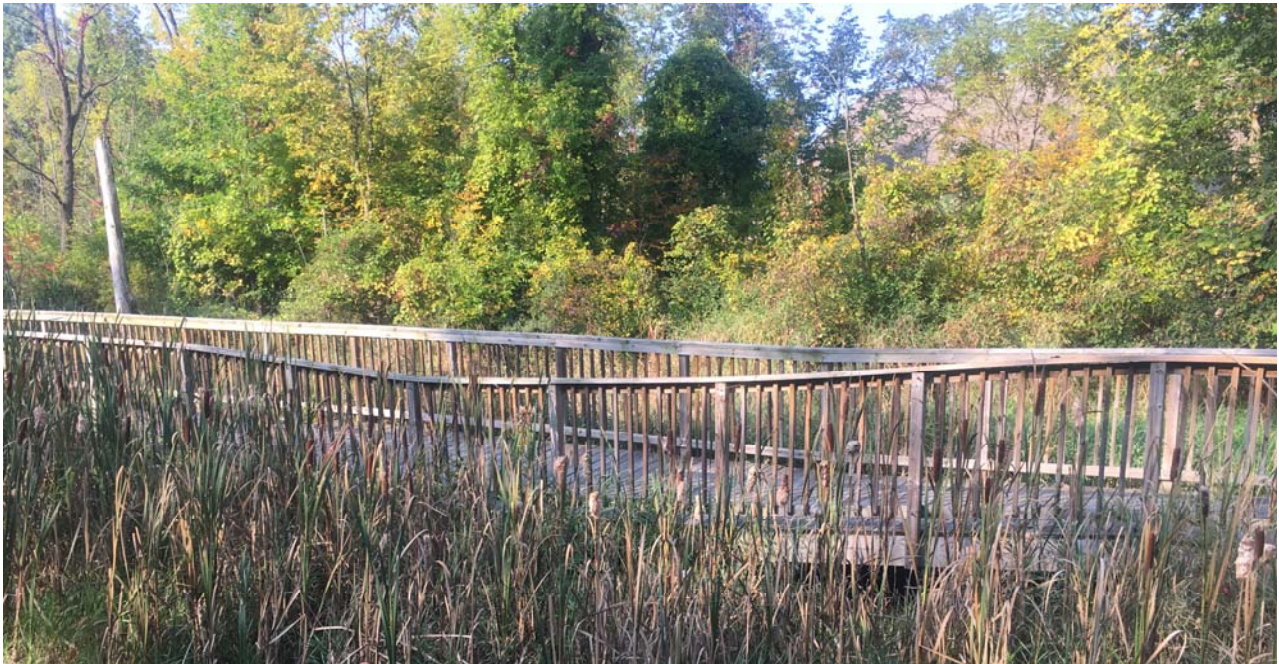
Boardwalk # 20: Unsafe boardwalk, located west side Beck, north of Cider Mill
