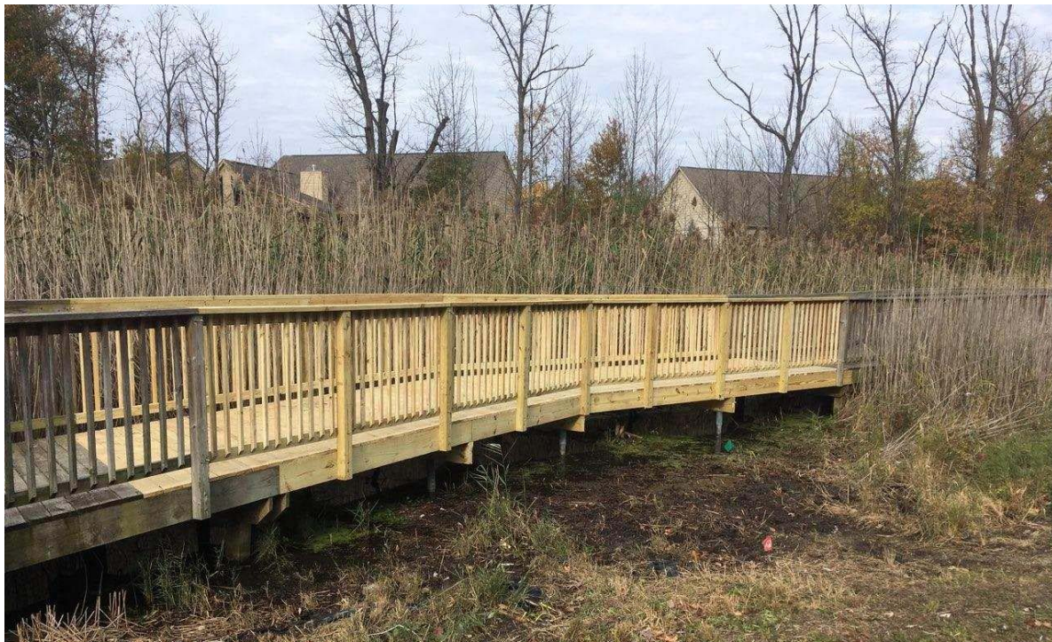
Beck Road Boardwalk - West Side of Beck & South of Kirkway Place (2018 Repair Project)
